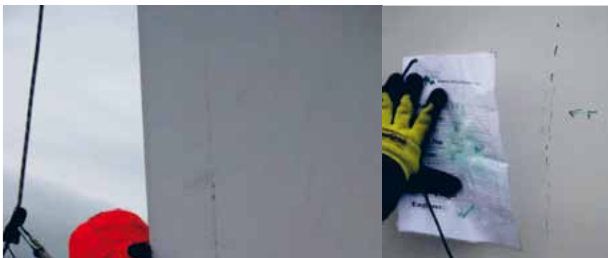
Fig. 4. Left: Crack near the trailing edge discovered by periodical inspection from a Danish major offshore park. Right: Crack near the webs.
